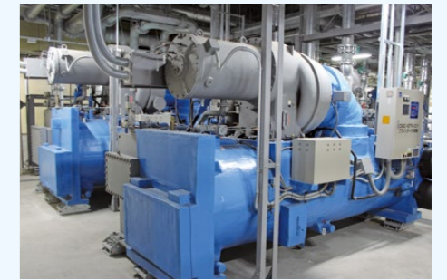
Chiller installed at the Kabukiza Theatre in Ginza, Tokyo
