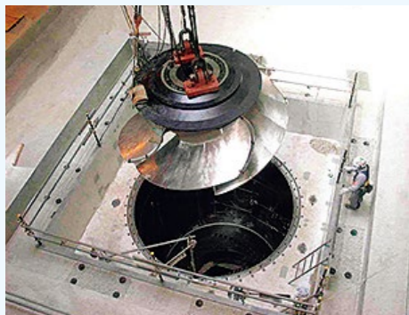
One of the world's largest drainage pumps installed in a flood bypass on the outskirts of the Tokyo metropolitan area
