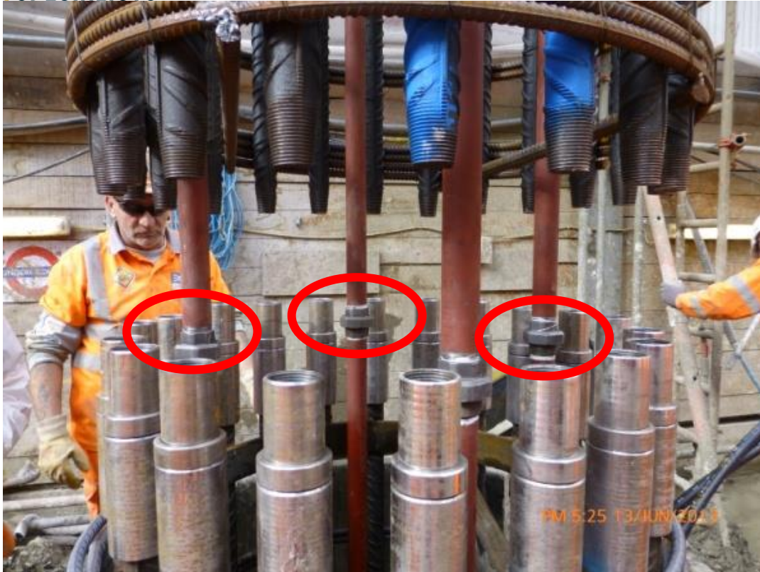
Figure 39: Union couplers connected within cage
