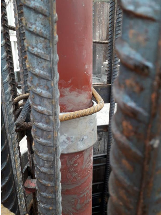
Figure 28: Stirrup obstructing the movement of the sonic point due to presence of tube joint
