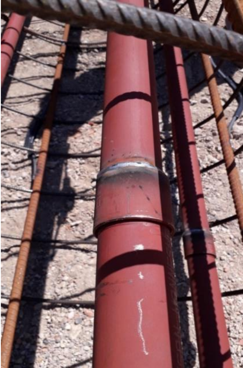
Figure 41: Joint detail for thick wall steel tube within one cage section (done by cage manufacturer)
