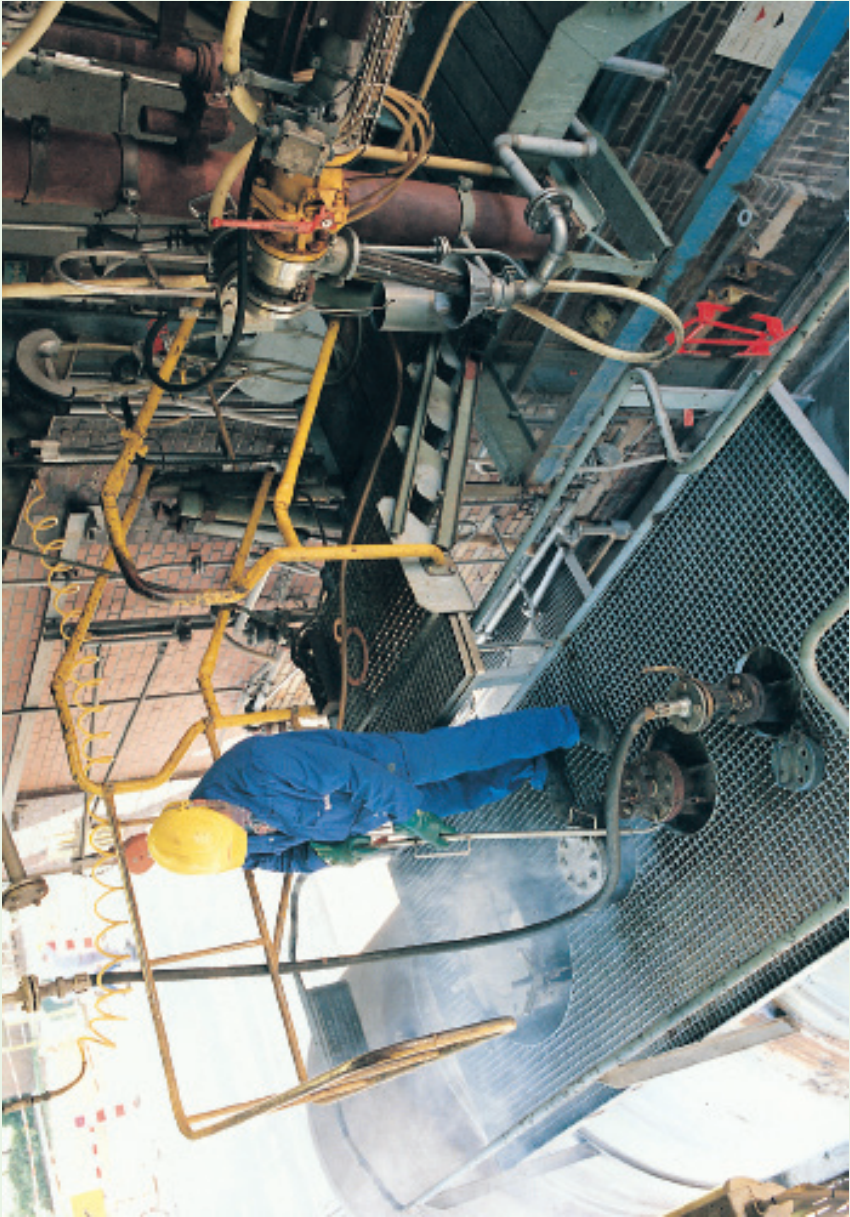
Fig 5 Demonstration of detection of a leak using a leak detector spray or ammonia; after pressure relief via the pressure nozzle, the blind lid is attached to the pressure nozzle.
