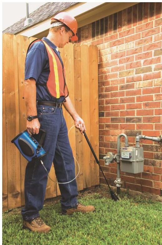
Figure IV-6: Checking a Gas Meter For Leaks With a Hand-Carried Infrared Optical Instrument.
