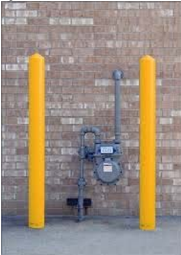
Figure VII-1: Outside Gas Meter with Vehicular Damage Protection
