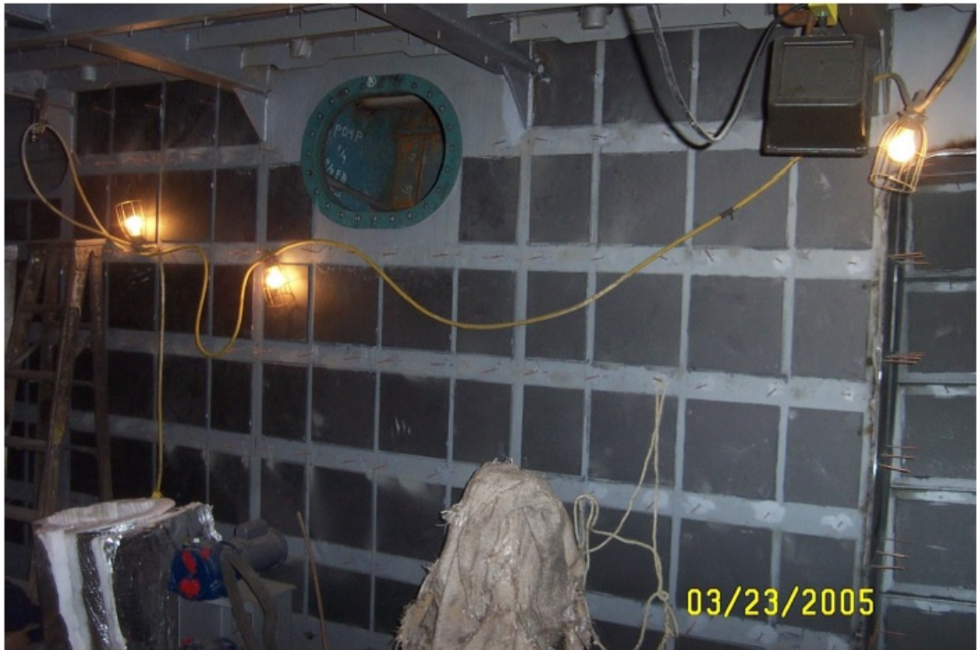
FIGURE 4 Unconstrained Tile Damping Applied to Hull Side
