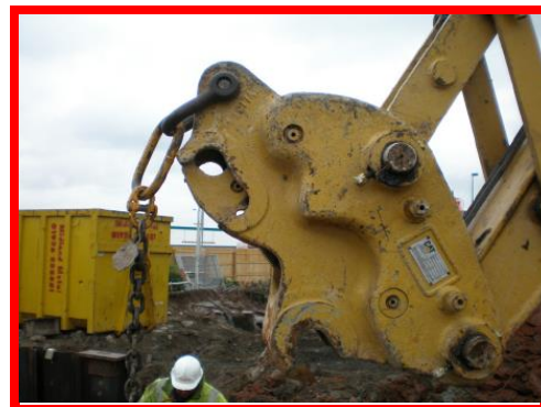
Figure 15. – Hitch tilted backwards with master link subject to twisting
