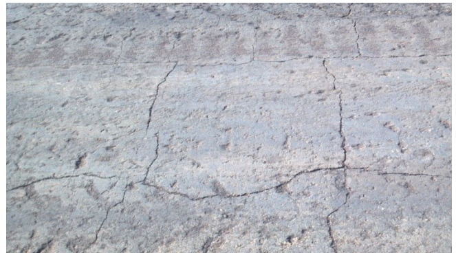
Figure 3.10. Block cracking on a compacted CTB layer
