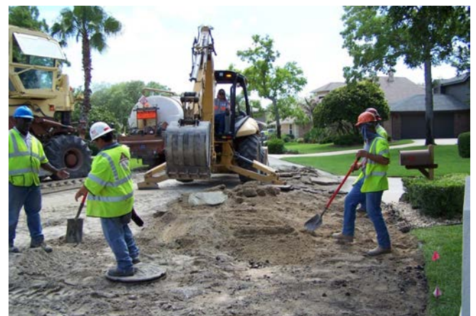
Figure 1.7. Utilities like this manhole may need to be lowered beneath the proposed FDR depth before construction
