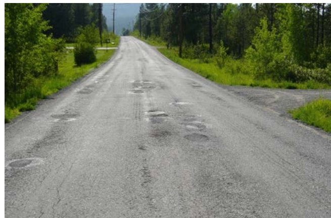
Figure 3.1. Excessive patching on asphalt roadway
