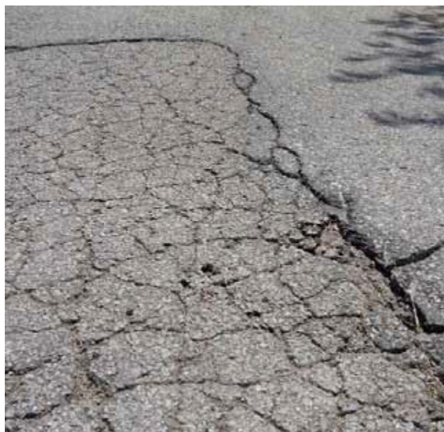
Figure 3.7. High-severity alligator cracking
