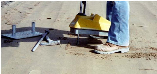
Figure 7.6. Density of compacted FDR being determined by a nuclear gauge in direct transmission mode
