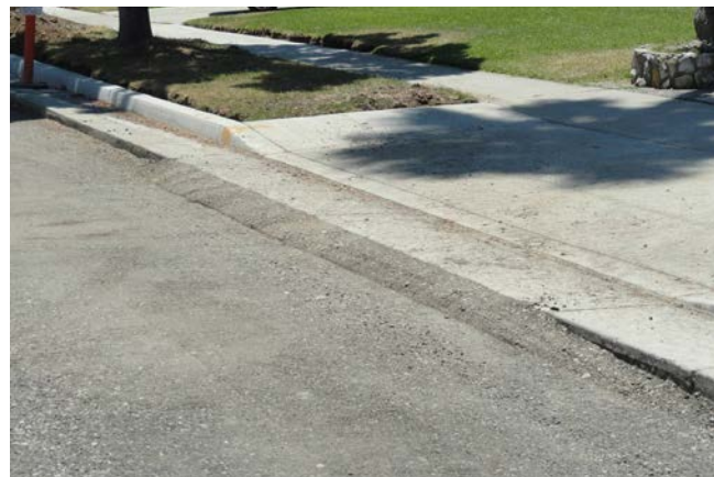
Figure 1.16. This compacted FDR base was opened to light residential traffic before application of surface course
