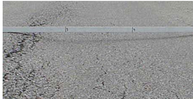
Figure 3.13. Low- to medium-severity rutting
