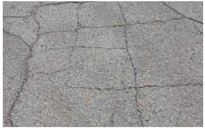
Figure 3.8. Low- to medium-severity block cracking
