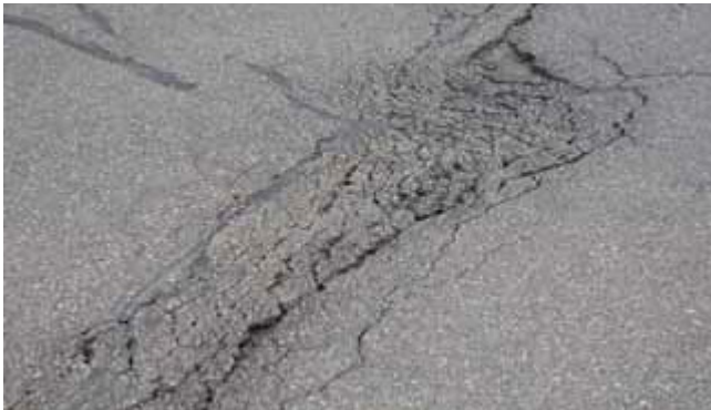
Figure 3.11. Low- to medium-severity pothole
