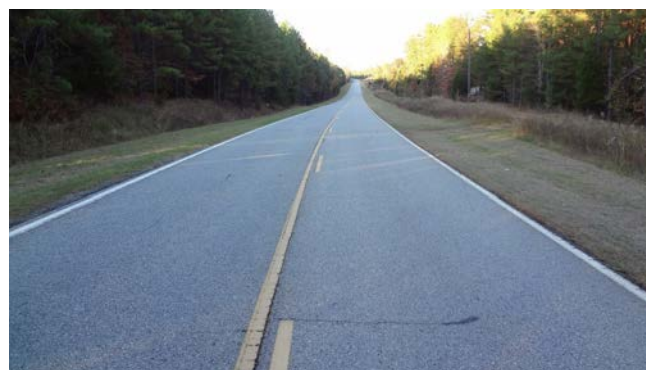
Figure 8.1. South Carolina state highway 97 (SC 97) is an FDR with cement project with excellent performance after 20 years of service
