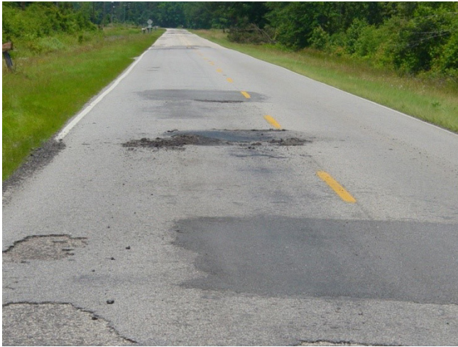
Figure 1.5. Asphalt pavement with patching
