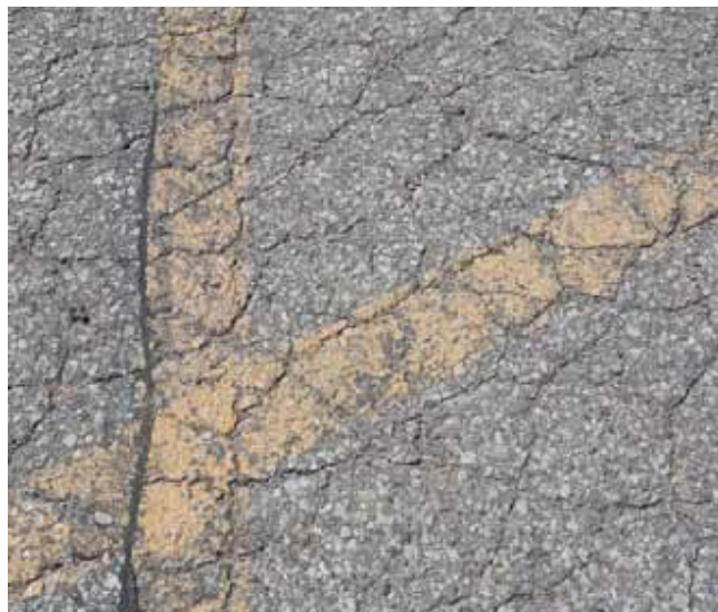
Figure 3.6. Low- to medium-severity alligator cracking
