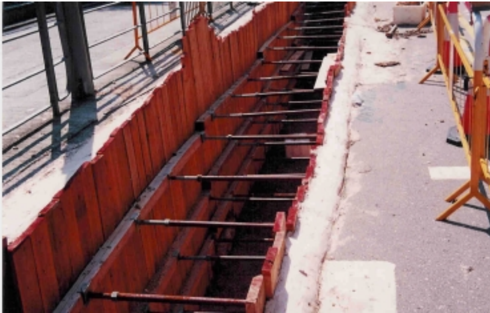
Plate B5 – Timber support protruding above ground with cement mortar wedge applied to prevent surface runoff
