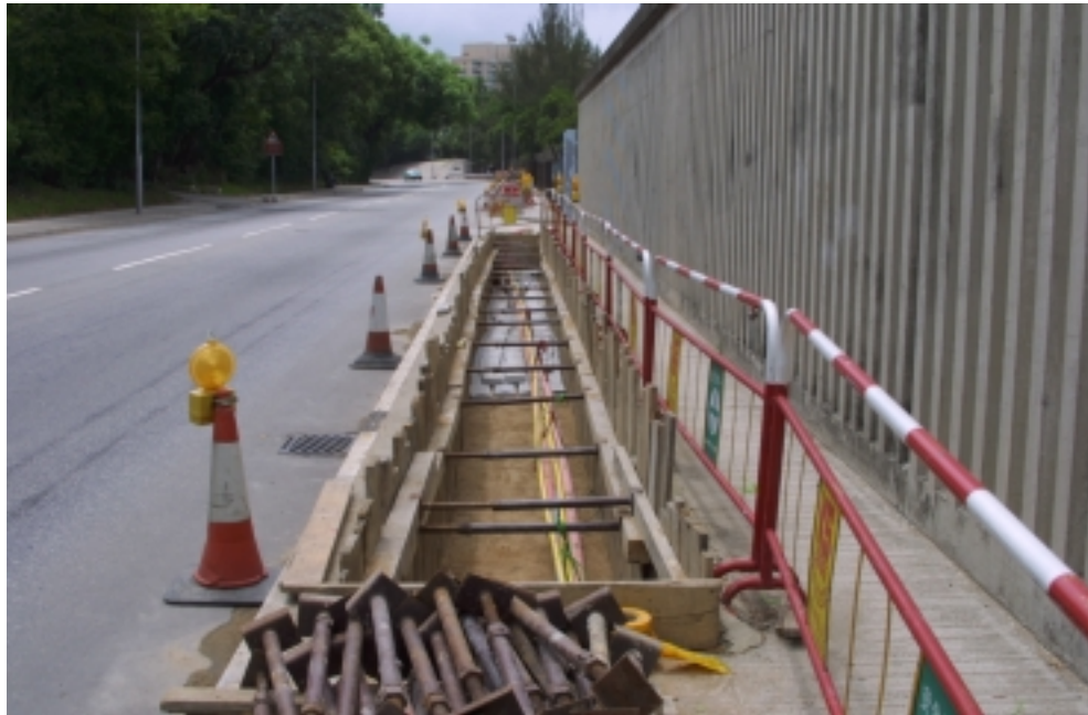
Plate A1 – Timber support with one layer of struts for shallow depth of excavation
