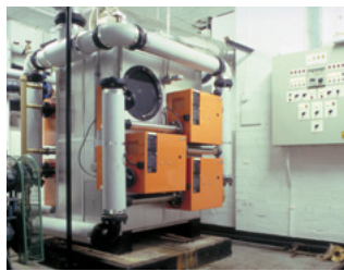
Image 26: Industrial heating, refrigeration and ventilation systems
