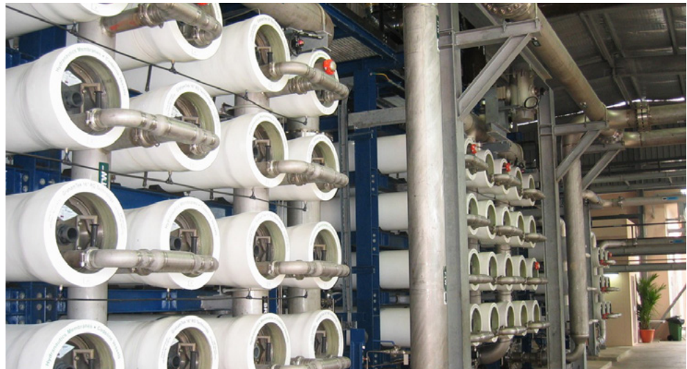
Image 5: Industrial scale seawater desalination plant
