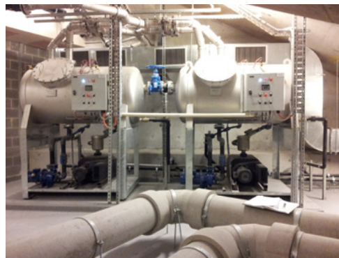
Image 3 (left): Closet of vacuum toilet system.
