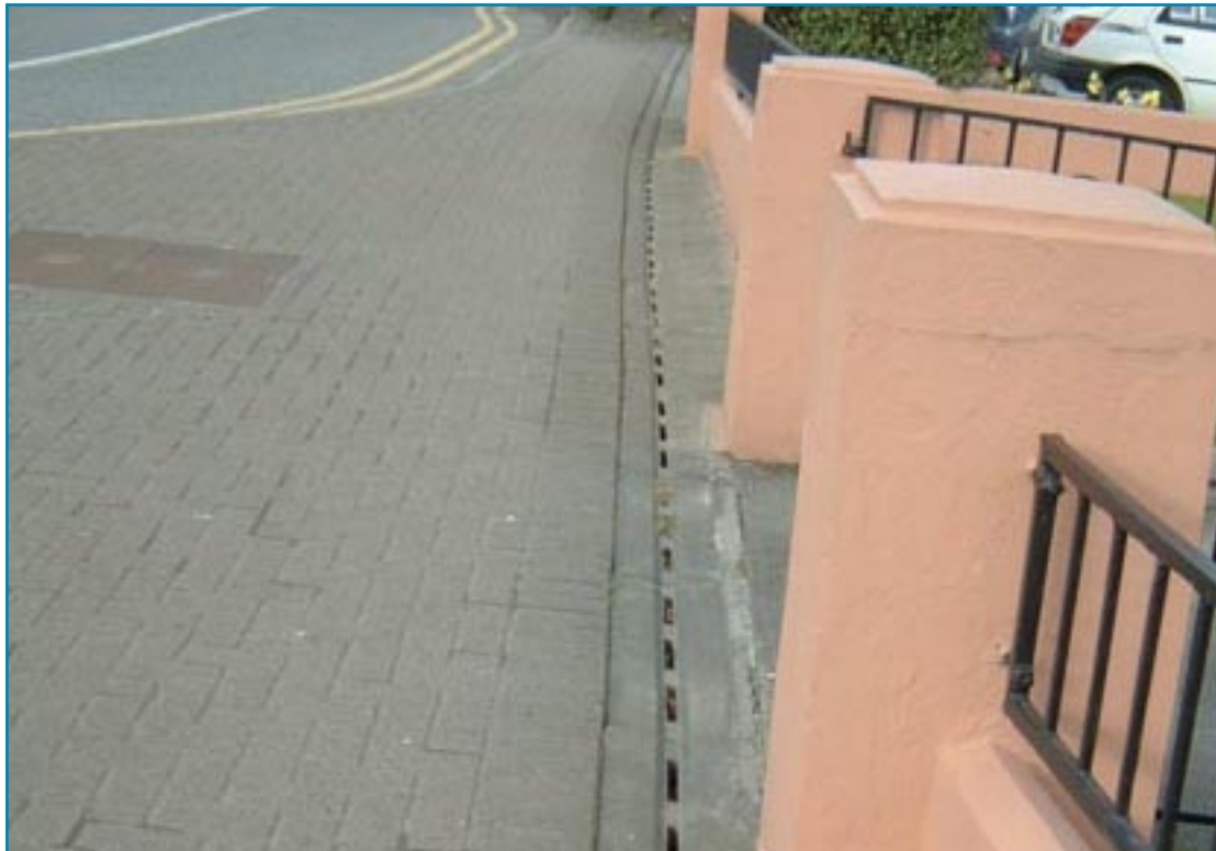
Photo 4.4 Linear Drainage Channel
