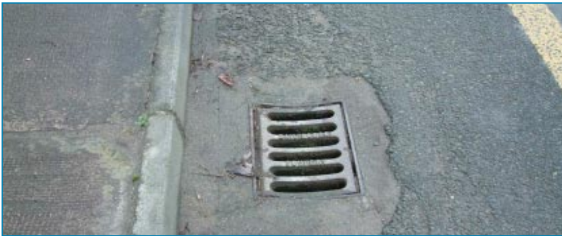
Photo 3.1 Gully is too far from kerb
