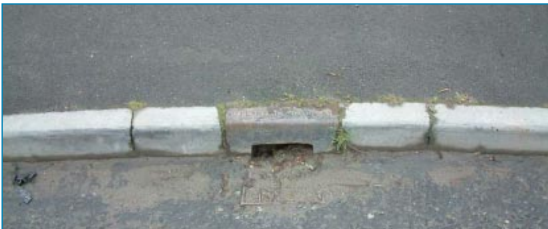
Photo 3.2 Poor Maintenance – Grating is barely visible
