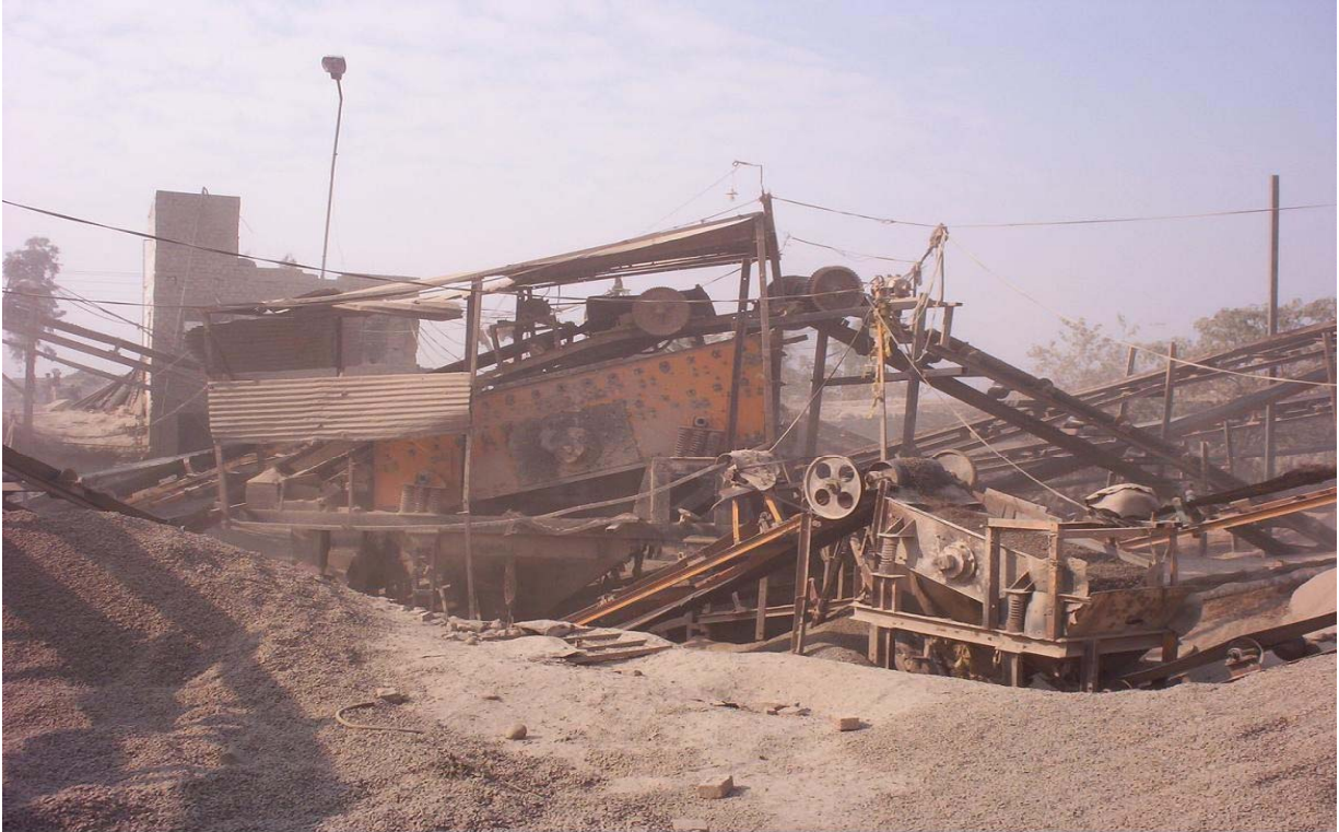
GENERAL VIEW OF CRUSHER
