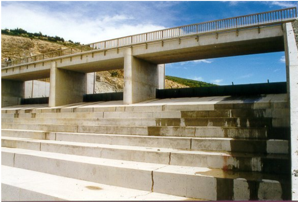
Figure 9: Ohuha Dam, New Zealand. Obermeyer adjustable flap gates installed on existing crest.
