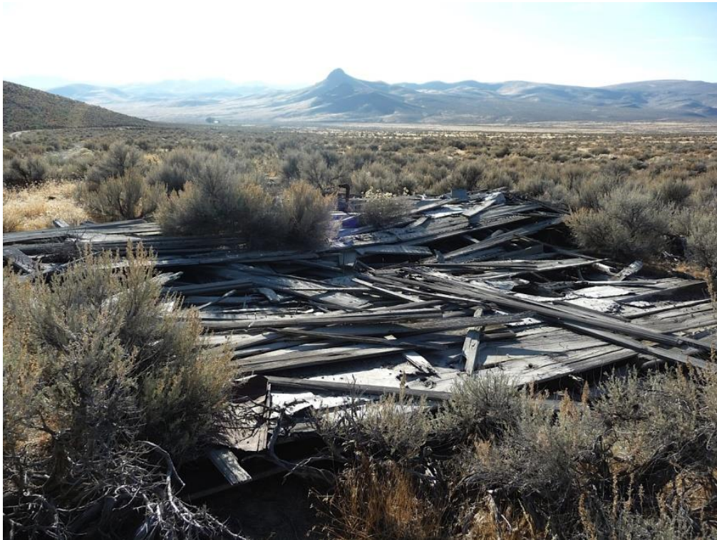
Figure 16: Use IMACS example: The floor and lumber from the collapsed walls is all that remains of this former building in Packard, Pershing County. (E. Dickey, 2012)
