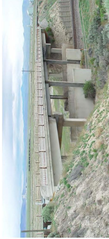
Moderne bridges, like this on ein Dunphy, Eureka County, were a standard design in Nevada in the 1940s. (Cliff Creger, 2011)
