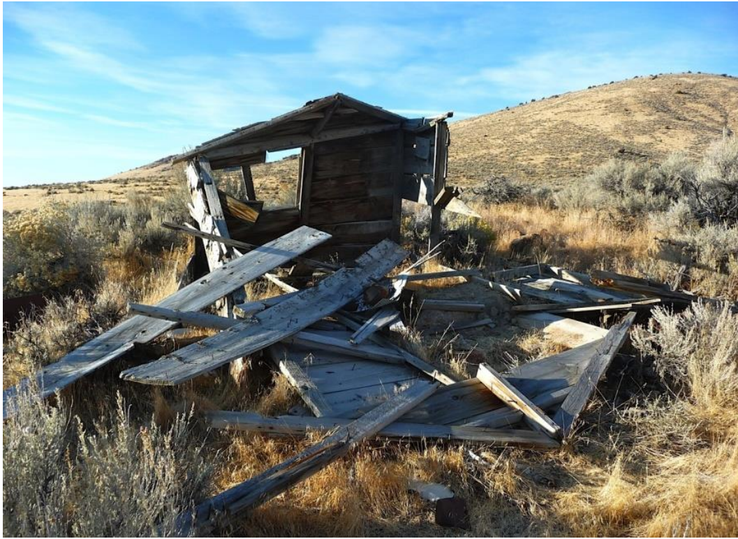
Figure 15: Use NARA form: This resource retains most of its elements, the walls, floor, and parts of the roof are still there, it has just fallen apart. All the elements of the building can be described and should be recorded on a NARA form. Packard, Pershing County (E. Dickey, 2012).
