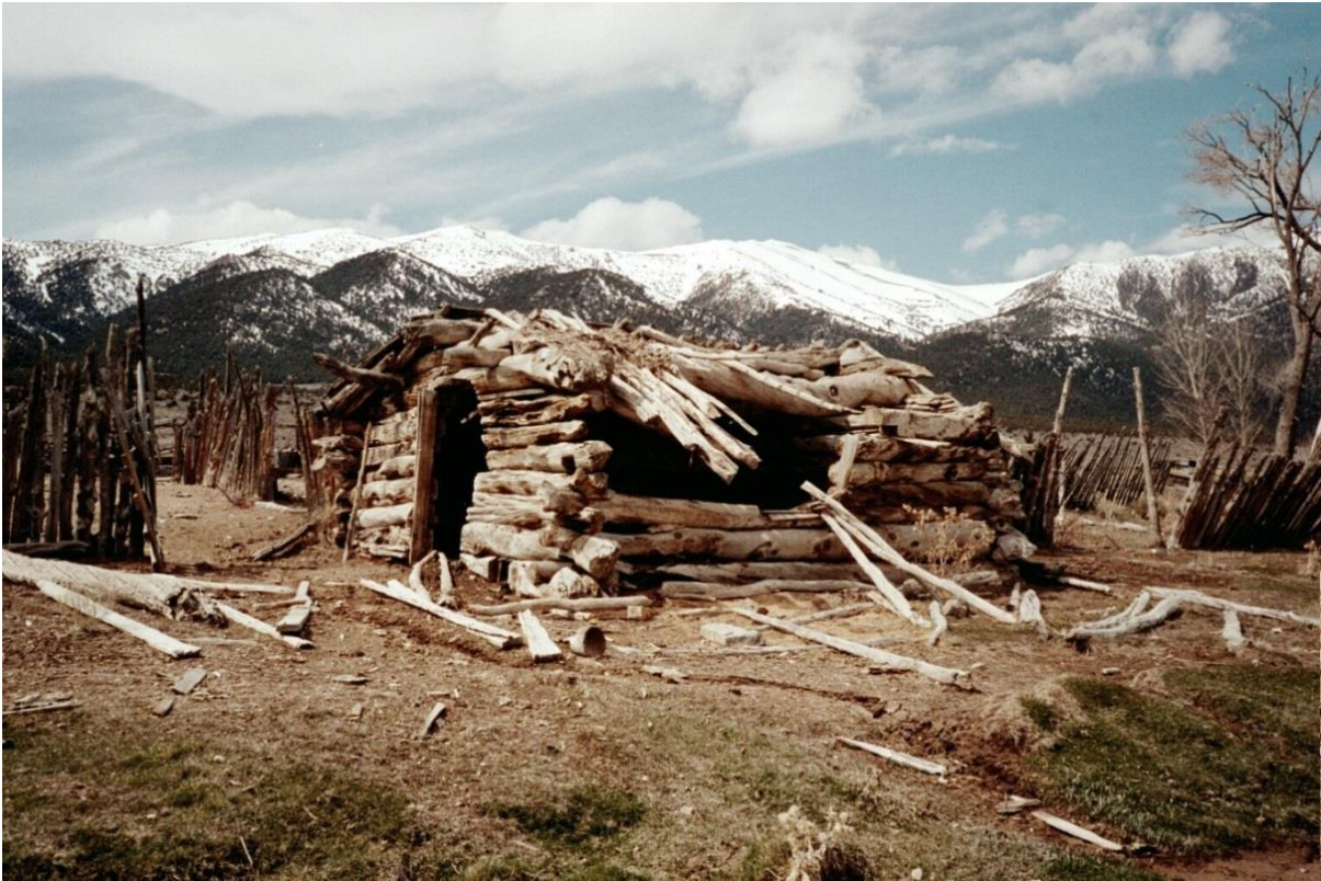
Figure 19. Cabin in poor condition, but with good integrity, Ruby Lake NWR (USFWS).
