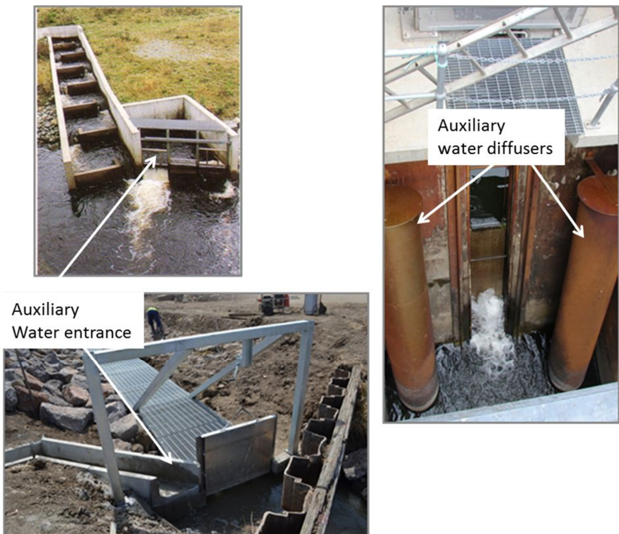
Figure 2.5: Auxiliary water systems for providing extra fish-attracting water adjacent to a fishway entrance: overfall weir (top left); small culvert (bottom left); and twin vertical diffusers (right). (photos: I. Stuart)
