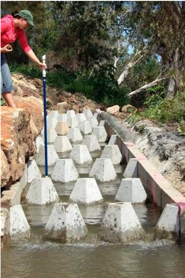
Figure A1.8: A cone fishway in Queensland.
