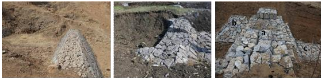
Figure 10. Gabion check dam with step body without an overfall outlet ( left ), double overfall outlets and riprap ( middle ), and footpath with a cement cover ( right ) ( a , spillway; b , revetment; c , apron extension) (left, middle, and right photos taken by Dr. X.Y. Zhang in June 2018, Fuxin City; in July 2018, Kaiyuan City; and in April 2018, Fushun County, Liaoning Province).
