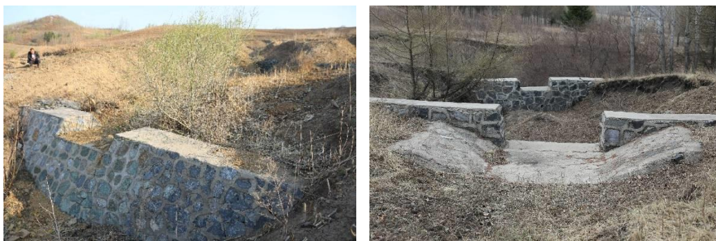
Figure 9. Rectangle type masonry check dam with cement surface (left) and masonry check dam supplement drop structure (right) (photos taken by Dr. X.Y. Zhang in April 2018, Liuhe County and Dongliao County, Jilin Province).
