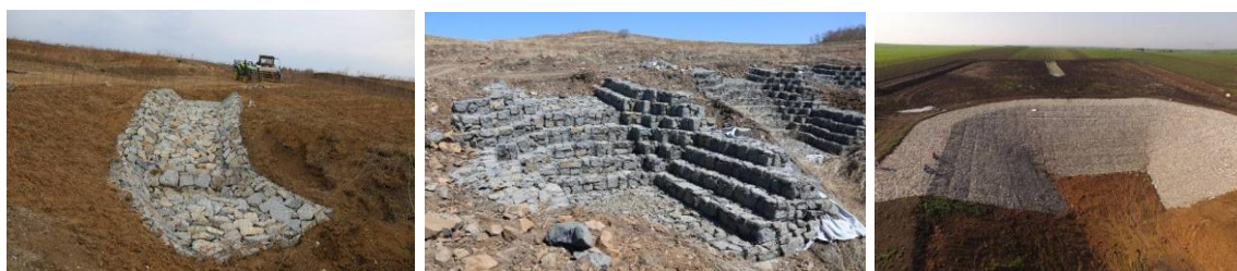
Figure 6. Drop structures with small-sized gabion ( left ), medium-sized gabion ( middle ), and large-sized gabion ( right ) (left and middle photos taken by Dr. X.Y. Zhang in April 2018, Dunhua City, Jilin Province; right photo taken by Dr. H. Li in June 2016, Hailun City, Heilongjiang Province).
