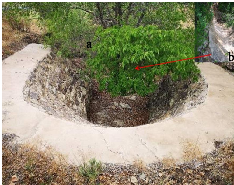
Figure 4. Arc-reinforced concrete and arc-concentrated and diversion masonry drop structure (photo taken by Dr. X.Y. Zhang in July 2018, Wulanhaote City, Inner Mongolia Autonomous Region).
