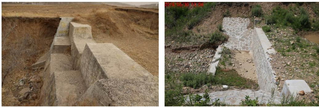
Figure 8. Step (left) and inverted trapezoid (right) type masonry check dam with cement surface (photos taken by Dr. X.Y. Zhang in May 2018, Zhangwu County, Liaoning Province and in August 2018, Hailin City, Hielongjiang Province).
