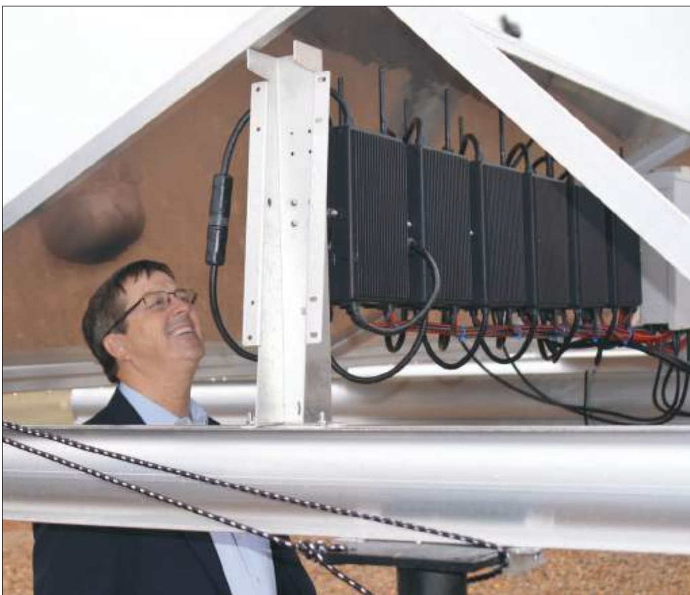
CLOSER INSPECTION. Senator Larry Teague of Nashville gets a closer look at the solar panels Wednesday morning at the 4-acre facility which turns sun rays into electricity at the Husqvarna plant north of Nashville.
