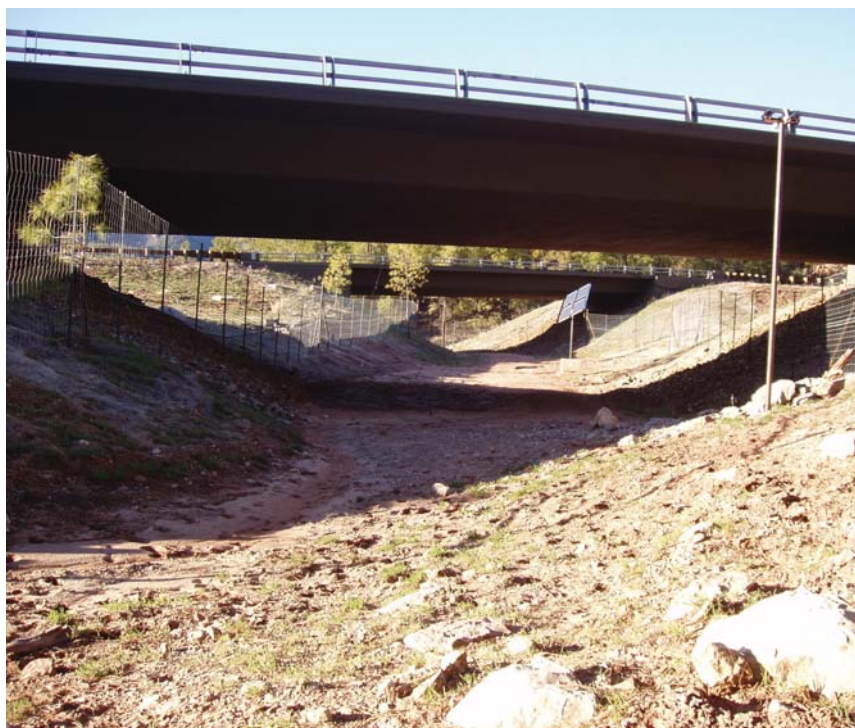
Figure 37. Highway underpass fenced to direct deer safely under the vehicle traffic. (Photo by Norris Dodd/AGFD).
