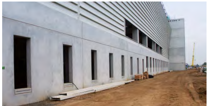
UPS Air Hub, Cologne Bonn Airport, Germany
