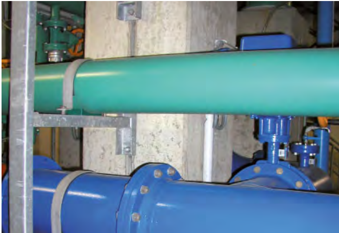
Pipe supports on vertical HZA Channels
