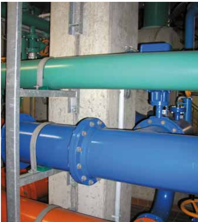
Pipe support using vertical cast-in channels
