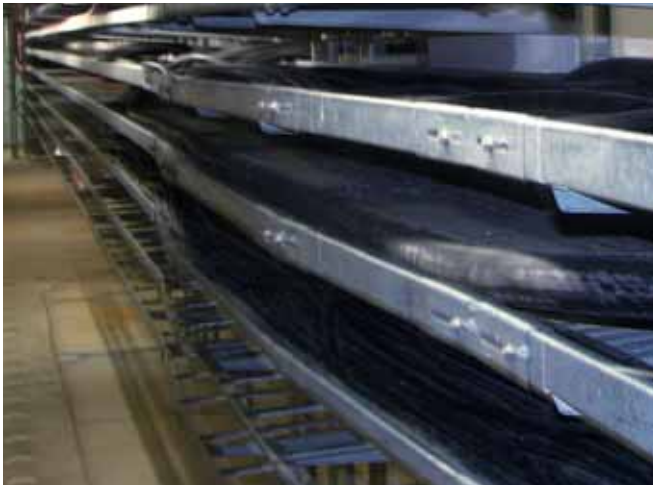
Stacked cable trays; by bolting to vertical serrated channels
