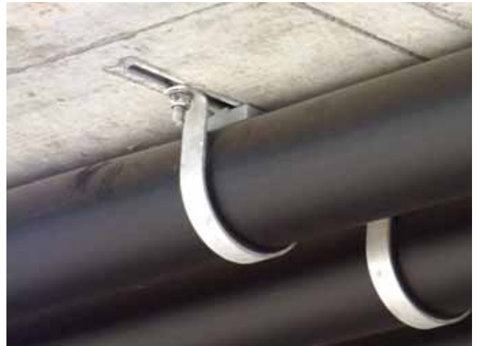
Pipe support bolted to ceiling
