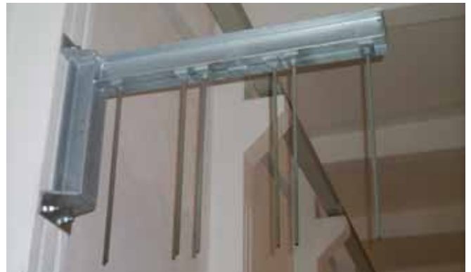
Cantilever for support of pipes mounted to vertical serrated channel
