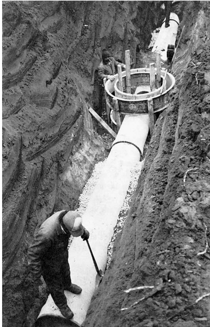
Fig. 12.12 Sewer pipe laid through and beyond manhole location prior to construction of manhole.
