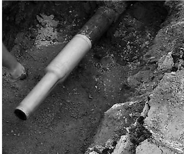
Fig. 13.15 Expanded structural liner with hardware removed.
