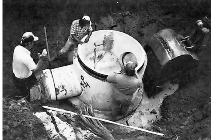
Fig. 12.16 Placing a gasketed pipe joint within 3 ft of each side of the manhole helps to accommodate possible manhole settlement.
