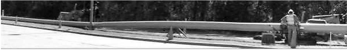
Fig. 13.7 PVC pipe supported on rollers.
