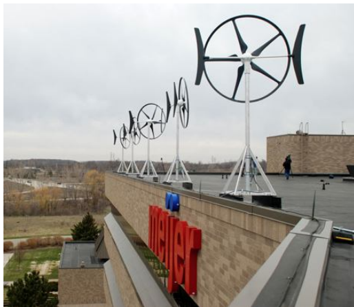
Image 1 -- turbine installed on roof of a building
