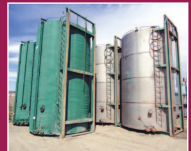
400 88L Storage Tanks
