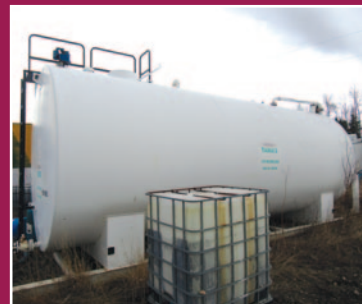
Fuel Storage Tank
