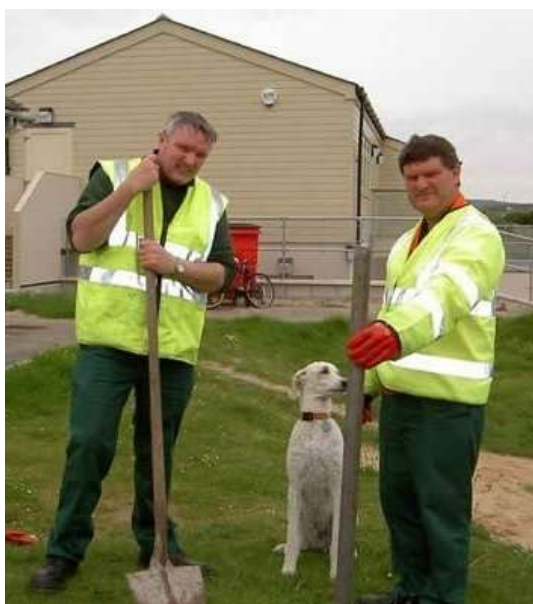
A 'CUSTOMER' WAITS ANXIOUSLY FOR A NEW DOG BIN TO BE INSTALLED.
