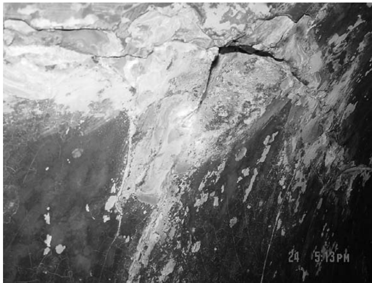
Figure 4. Close-up of interior mortar crack
