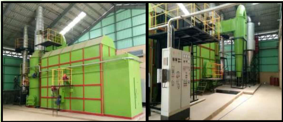
Gambar 1. Mesin Incinerator PT. Andhika Makmur Persada
