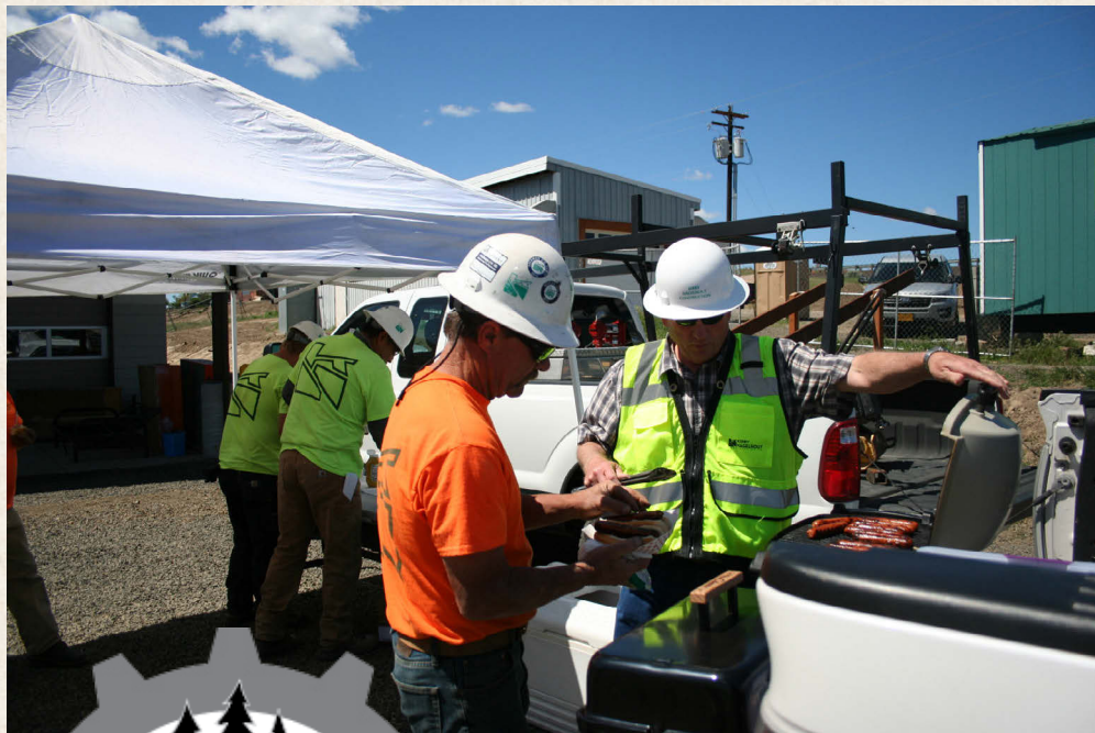
Kirby Nagelhout Construction in Bend held several Safety Break-related activities in 2016, including toolbox talks and barbecues.
