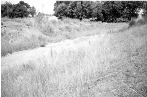
Poor coverage on upper slope
