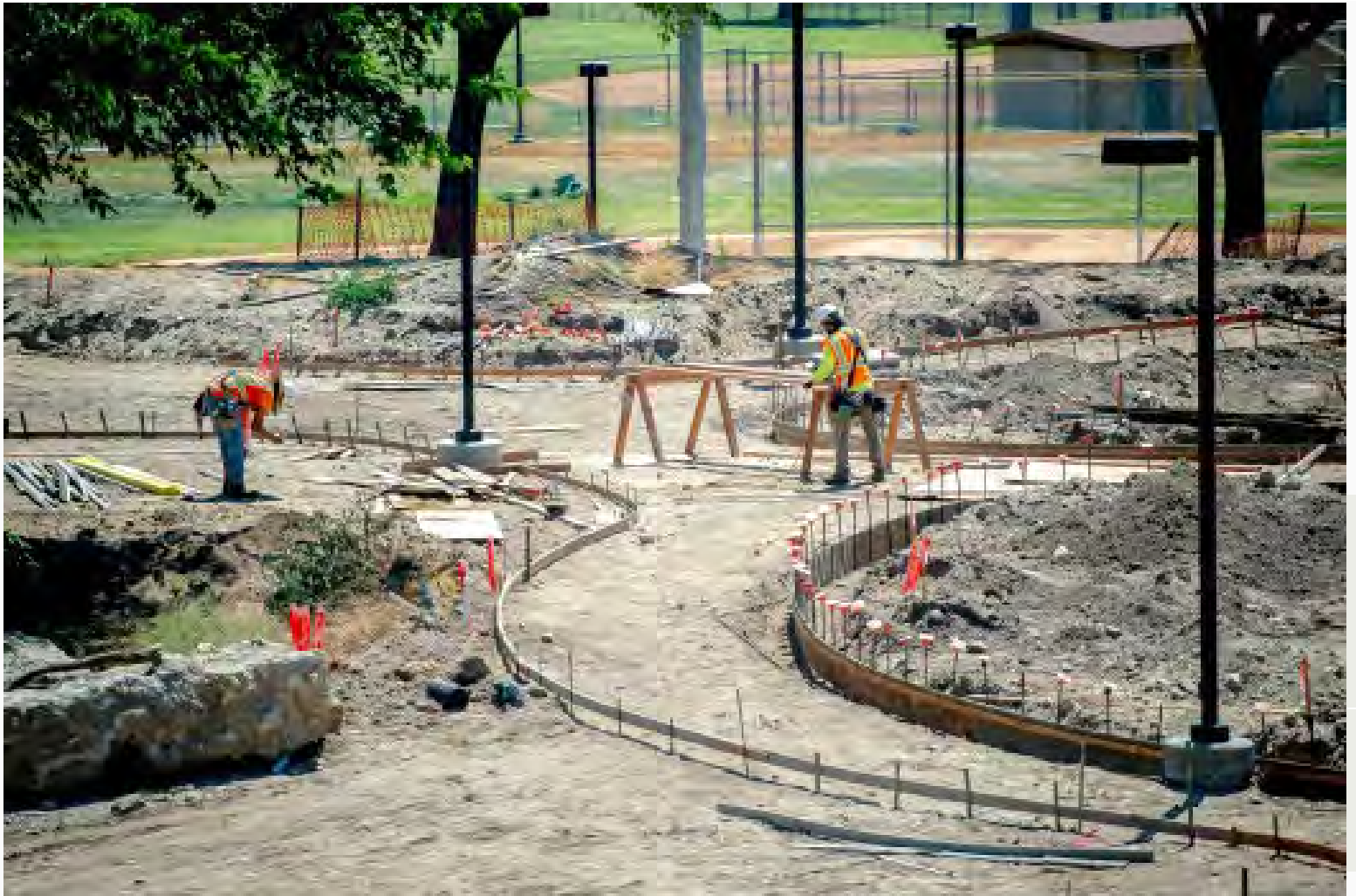
Construction crews work on the expansion project at Frisbie Park in Rialto on Tuesday, June 30, 2020. (Photo by Watchara Phomicinda, The Press-Enterprise/SCNG)
