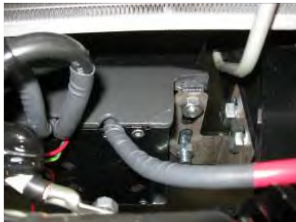
Figure 20: Control pack and Bracket Installation. (16.5Ti shown)
