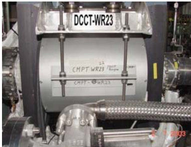
Figure 2: The HERA-p DCCT installation: a more complicated structure with heat sinks.
