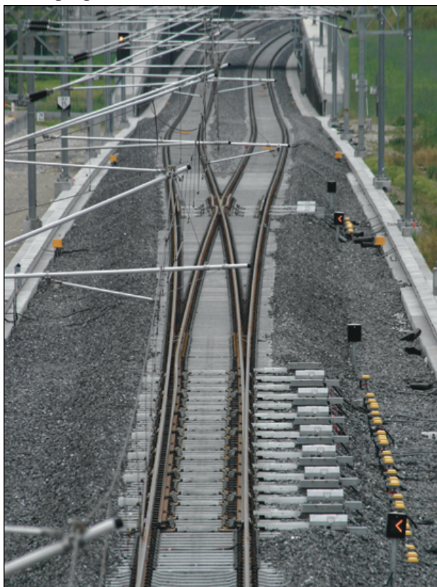
Figure 3: High speed turnout designed for 200km/h operation. The turnout is 164m long with 65m switch rails and 8 motors, plus an additional 3 motors for the movable crossing angles. Photo: Georg Trüb of Railpictures.net.
