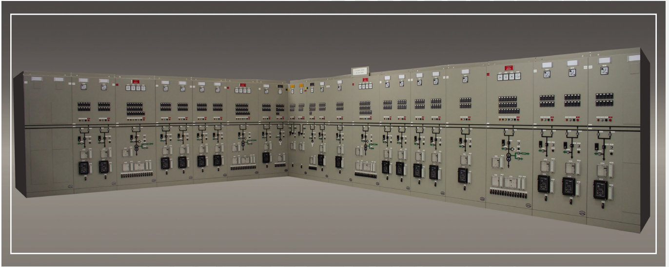
11kV Remote Control and Protection Board In 'L' formation
