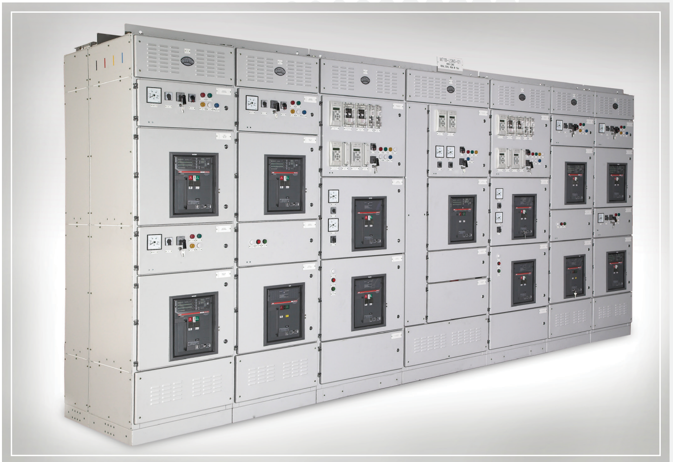
Main Low Tension Board
