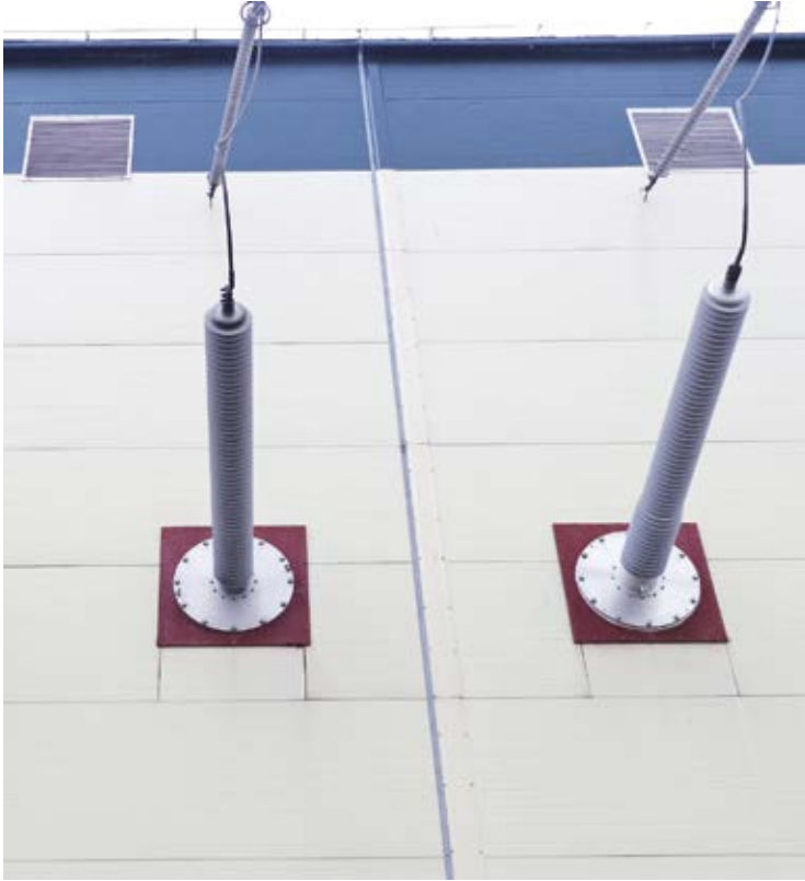
Wall bushings 252 kV produced by Izolyator company on the switchgear of an oil-processing plant
