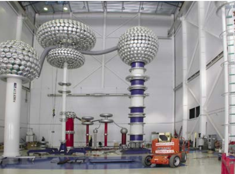
Fig. 14. Testing area for 252-1200 kV bushings at the Izolyator plant
