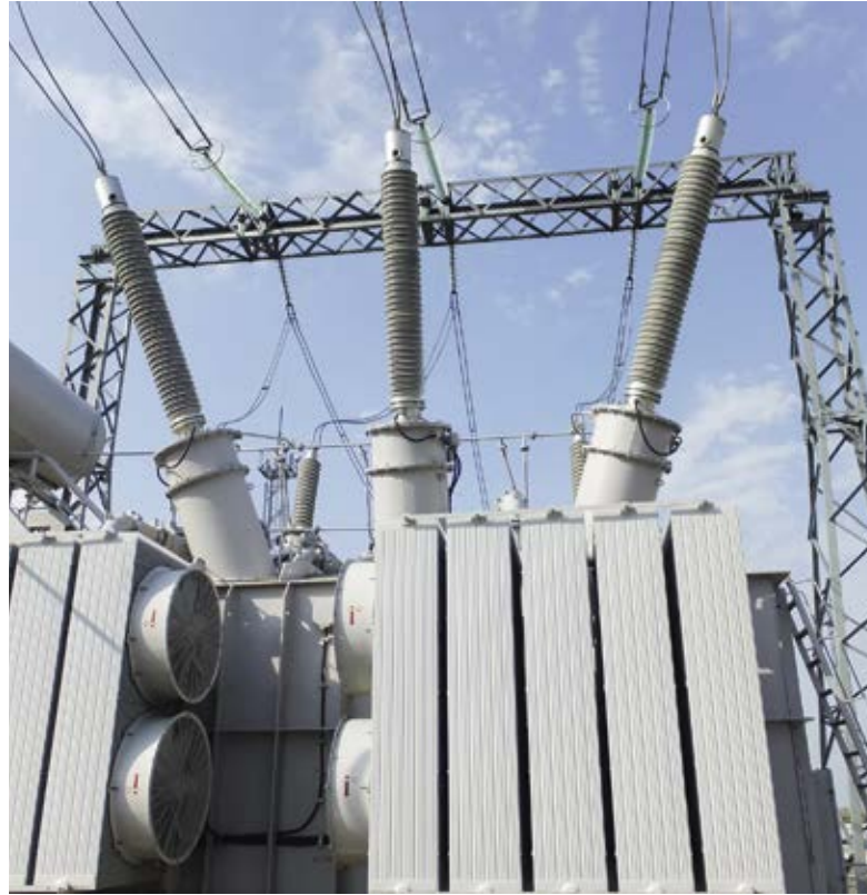
Bushings 363 kV produced by Izolyator company on the transformer of main power grids
