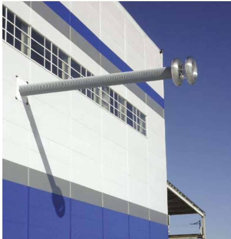
Line bushings 820 kV DC at the testing center of Izolyator factory
