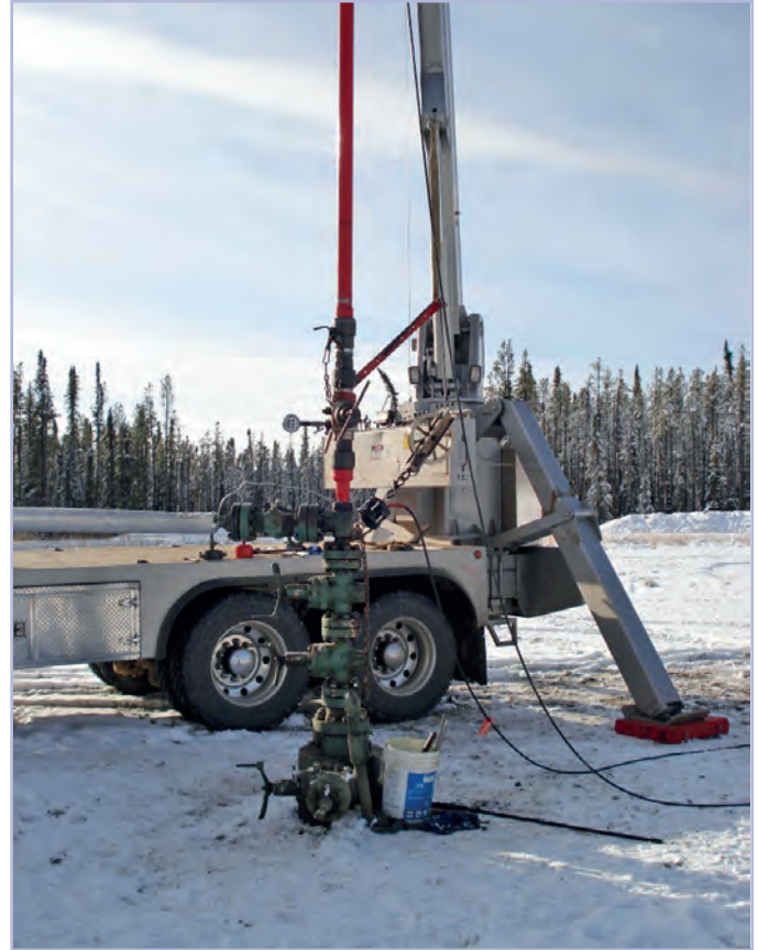
Figure 4: Wireline attached to the top of a Christmas Tree
