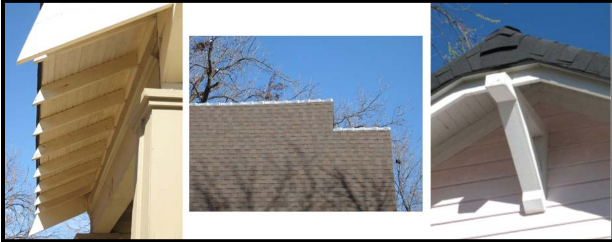
FIGURE 36: PRESERVE ORIGINAL ROOF FEATURES, SUCH AS EXPOSED RAFTER TAILS, RIDGE TILES AND SUPPORT BRACKETS. meet the Guidelines for materials and location is not subject to review and does not require a Certificate of Appropriateness (for repair, replacement or installation of historic roof features, see Administrative Review).
