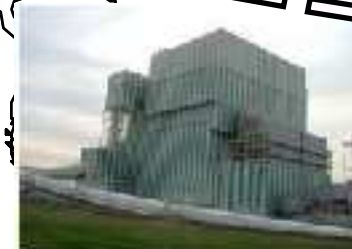
Japan, TEPCO/ Hitachi Naka No.1 1000MW, Coal
