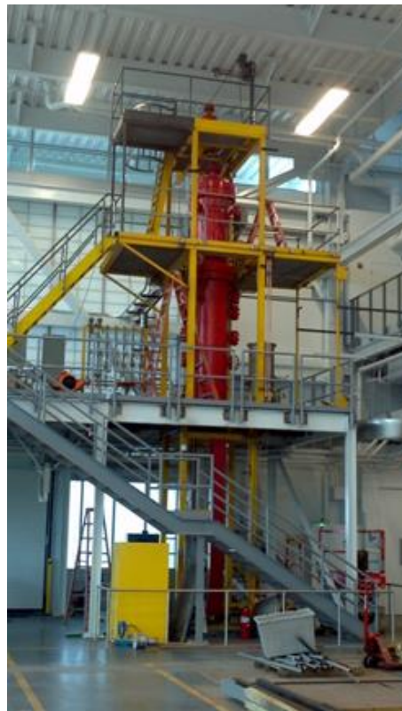
The IPST/ GA Tech Pressurized Entrained Flow Reactor in the high bay at C-NES.
