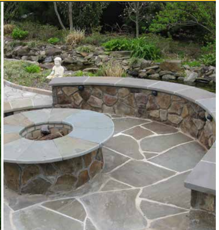
HOLLOWAY FIELDSTONE VENEER BENCH, MORTAR JOINTS AND LED LIGHTING. IRREGULAR FLAGSTONE PATIO AND FULL MASONRY FIRE PIT.
