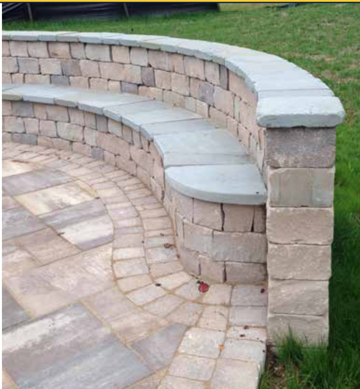
CHAPEL STONE SEATING WALL AND BACK REST WITH TUMBLED FLAGSTONE CAPS. CAMBRIDGE XL PAVER AND HANOVER TUMBLED BORDER .
