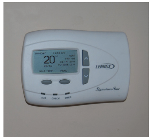
Figure 7: Lennox Signature Stat programmable thermostat at the house
