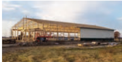
2019 begins a new chapter for Cattle Visions as we start construction on a building to collect and house bulls. We are "at your service!"
