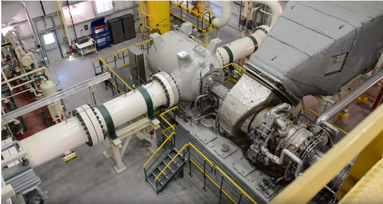
Solar Titan 250 and gas compressor at a Spectra Energy gas compression station.
