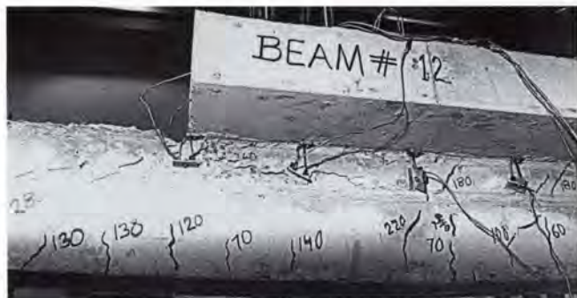
(a) Local crushing and the crack path through the web.
