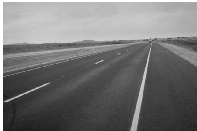
FIGURE 19-7 Asphalt bleeding in travel lane.
