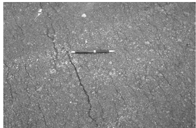
FIGURE 19-4 Hairline cracks caused by roller checking.
