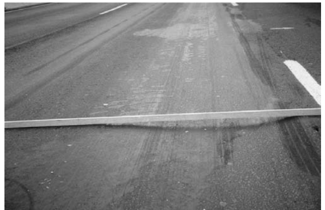
FIGURE 19-6 Rutting of unstable asphalt mixture.
