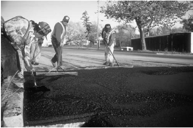
FIGURE 17-7 Excessive raking of transverse joint.
