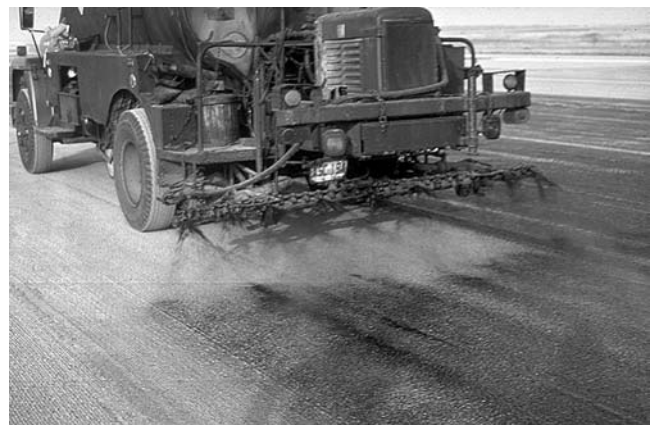
FIGURE 14-8 Improperly adjusted distributor.
