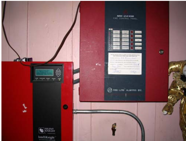
Alarm Panels should be inspected to confirm that the system is operational.
