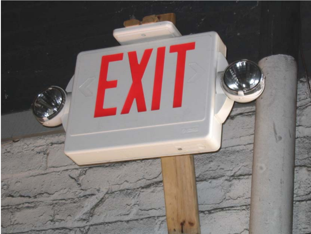
Indicator lights on self contained emergency light units will reveal the status of the back-up battery. Some units have a test switch.
