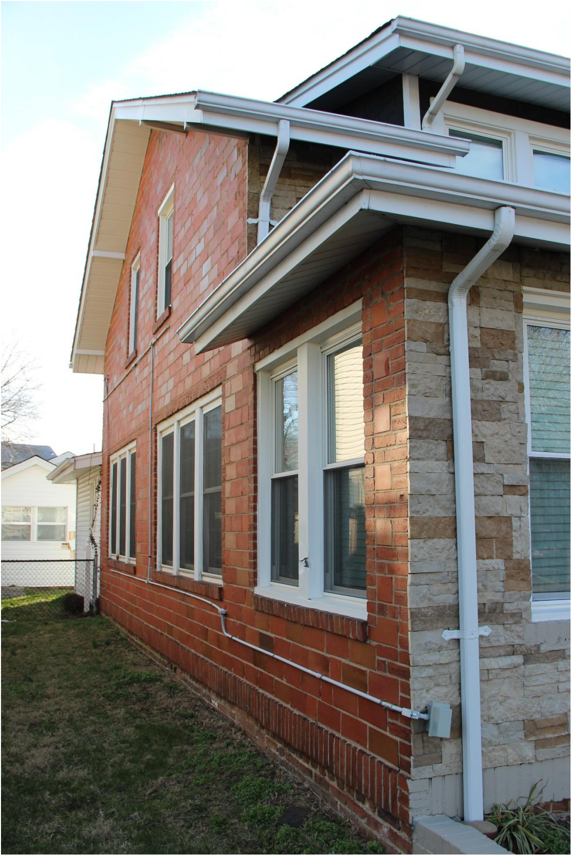
Figure 4: View of the north elevation from the front yard. Photograph by Kyle Fisher, March, 2018
