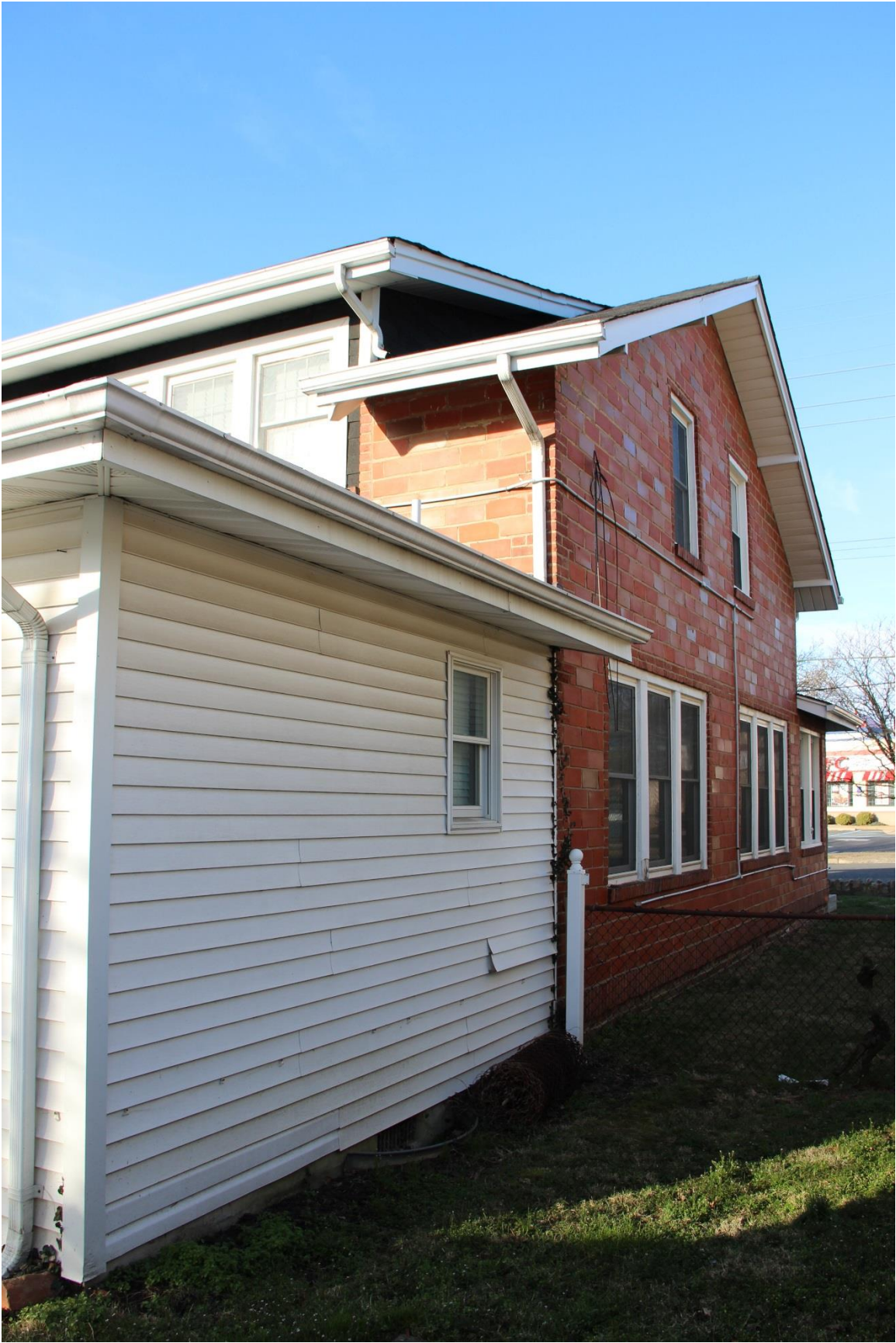
Figure 3: View of the north elevation from the rear yard. Photograph by Kyle Fisher, March, 2018
