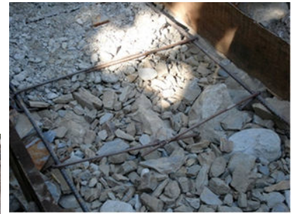
Figure 3 6. RC plinth band under construction (note poor splicing of stirrups) (Note: This was constructed for ERRA reinforced masonry. Picture was taken in Leepa in September 2006 before dhajji decision from ERRA. Picture from an area with no prior knowledge of reinforced concrete construction.)
