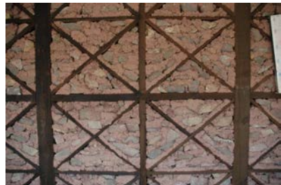
Figure 3 39. Reasonably cut stone laid with a lot of mud mortar. Note that the timber has been soaked in old engine oil as a way to give it some better protection against rotting.
