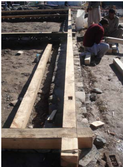
Figure 3 47. Base plate corner detail and bolt anchorage holes. Note that orthogonal walls are already planed and interconnected with the perimeter timber ring beam.
