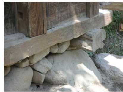
Figure 3 3. Foundation below plinth beam, note no connection between plinth wall and timber beam (existing building).
