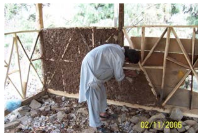
Figure 6 8. Infill construction from stone, mud and backing board that acts as temporary form work. Note: CGI as sometimes used for the form work these days and sometimes left then as permanent formwork/weather protection (used for this reason rather than to stiffen the frame). It is still the case that timber planks are most common.
