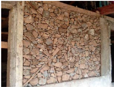
Figure 5 16. Mix of RC columns, dhajji infill construction (note the large panels of stone infill and limited amounts of timber bracing).
