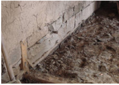
Figure 5 14. Timber sill beams and columns in direct contact with the ground exposing the timber to moisture. Note that the infill looks more like a dry stone wall.
