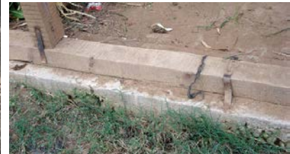
Figure 3 9. Timber ground beam (or sill beam) raised above the ground to protect the timber frame from rotting. Note attempted connection of the timber beam with the foundation. Damp proof course not provided.
