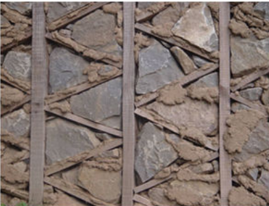
Figure 3 16. A completed wall, note large stones. (Note: This was built before the earthquake; it is a cheap commercial building. Mostly for houses people use smaller stones and are afraid of large stones falling on them. They may use chicken wire or timber boards to brace or line the upper few feet of the internal wall to restrain stones from falling.)
