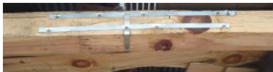
Figure 3 32. Strapping around the timber will help confine the scarf joint; long straps will help with tension as will the nails.
