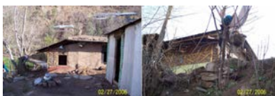
Figure 3 56. Single storey house with dhajji walls. It was not clear if the roof damage was due to the 2005 earthquake or if this was post earthquake construction. The exposed timber looked like post earthquake construction with fresh cut timber along the long facade.
