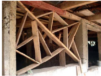
Figure 5 15. Mix of concrete columns with timber dhajji. Note poor quality compaction of the concrete and large cracks in the concrete column.
