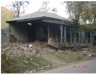
Figure 5 20. A building with dhajji in one direction, and stone URM wall in orthogonal direction
