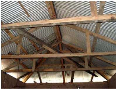
Figure 3 29. An internal view of a hipped roof. Apart from the CGI sheets there is no bracing to stiffen the roof structure. (Note: This roof is likely for storage/use. There will be a floor and ceiling of some kind added at a later date depending on the budget available.)
