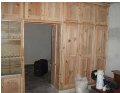
Figure 3 53. Full height built in wardrobe with reasonable thick solid timber back possibly it acts in part as a timber shear wall but it is not a detail that the engineering solution should depend upon. Note: The wardrobe back wall is usually solid 1/2 inch timber.
