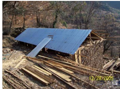
Figure 5 18. Dhajji house built into the hill side making the building act as a retaining wall. There is likely to be a stone wall at the back called a breast wall locally.
