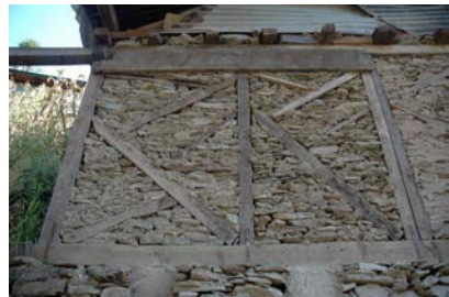
Figure 3 36. Bracing using large timber braces as timber resources are less constrained in the higher altitude. Note the more layered infill effect due to the type of locally available rock.
