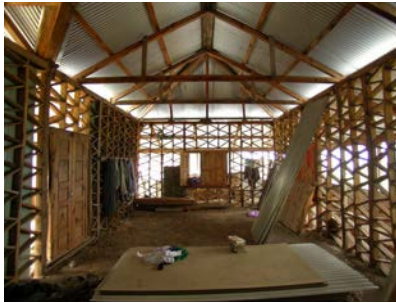
Figure 3 44. Inside view of a 1 storey house under construction. Note that the timber frame is in direct contact with the ground.
