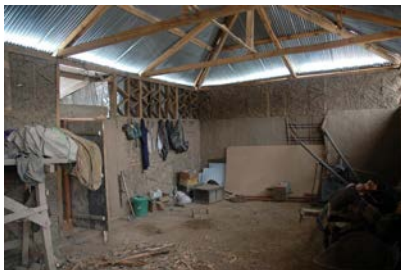
Figure 3 49. Internal view of large room with partially completed infill walls. Note the lack of bracing in any direction from the roof and apparently large distances between orthogonal walls. The system may be too flexible without enough support to the walls. There was some buttressing by walls of external rooms. This room is a hall for social occasions and shared use in winter, most families will not subdivide this room.
