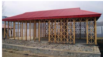
Figure 3 42. Zigzag bracing that nodes out. Note that the roof is erected early as it helps to stabilise the walls before their completion and helps keep the work dry. Also note the hipped roof giving stiffness in both principle building directions. Note 1: anchor rods in the foreground and that a damp proof course is not used. Note 2: The whole
