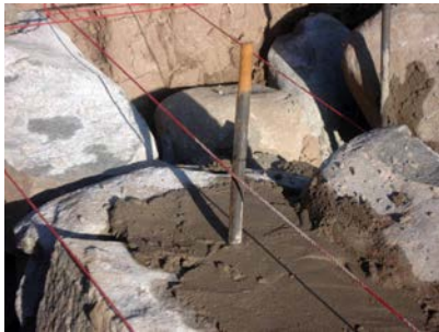
Figure 3 46. Anchor bolt in stone masonry wall laid in sand and cement mortar. Note that the mortar is only used locally around the anchor. Also note that the bolt is already rusting and is unlikely to receive any rust treatment prior to connecting to the frame base plate apart from being maybe treated with old engine oil which is very commonly done.
