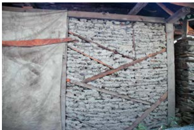
Figure 3 37. Large panel that appears to be in poor contact with the timber frame. Lack of tight fit may result in the entire panel falling out-of-plane. Again note the layering of the infill due to local rock characteristics.
