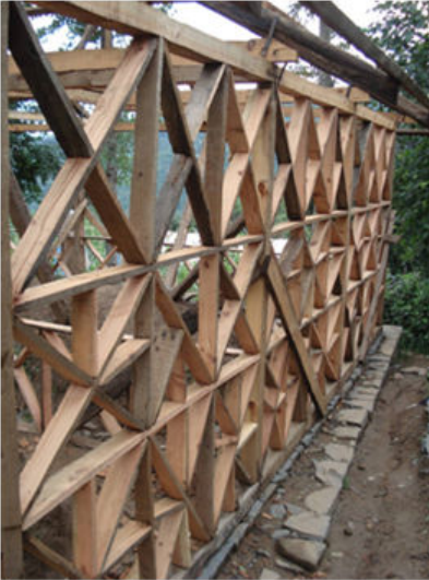
Figure 3 13. Timber frame ready to receive brick or stone infill, bracing is very much in the form of x-bracing.
