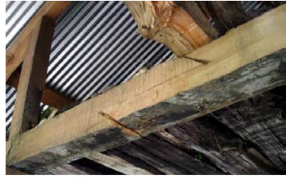
Figure 3 30. Timber connection details. Unless nails have been used this connection will not have very limited tension capacity to poor joint interlock.
