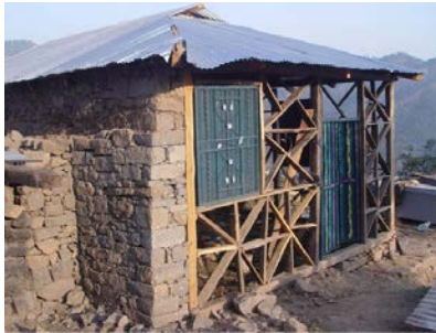
Figure 5 17. Dhajji in one direction and unreinforced stone masonry in other. Back wall of the house also acts as a retaining wall. It is not known if the wall perpendicular to the back wall of the house has buttresses to give it additional strength
