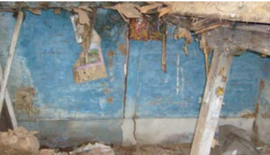
Figure 3 22. Close-up view of photograph in Figure 3 21, note post at mid room to support floor structure (Simla, India).
