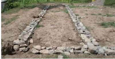
Figure 3 4. Stone strip footing under construction to raise the timber frame off the ground (new building).
