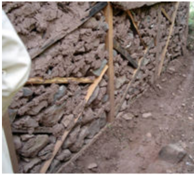
Figure 5 13. Timber frame that is not protected from moisture a major cause of timber rotting due to direct contact with the soil.
