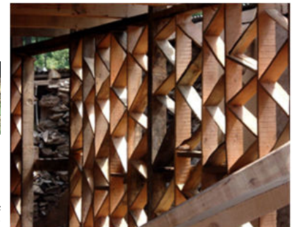
Figure 3 12. Timber frame ready to receive stone infill. Bracing has a zigzag pattern and bracing does not coincide/node-out.
