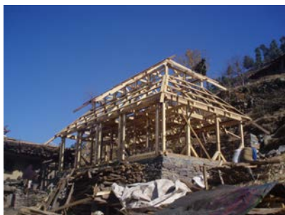
Figure 3 52. Dhajji frame under construction. Note that the front sits on top of a retaining wall and the back is partially a retaining wall. (Note: Front retaining walls are usually constructed too steep without the required inclines.)
