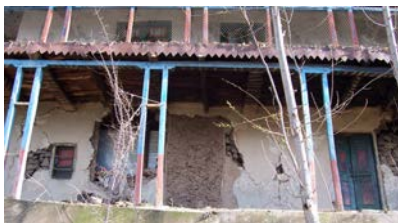
Figure 5 22. Dhajji wall intact apart from mud plaster that has fallen off. Plain stone masonry walls have partially failed, near Bagh, Pakistani Kashmir.
