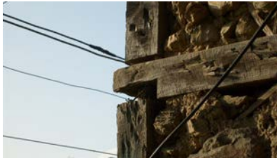
Figure 3 23. Connection of first storey post with second storey post with a cylindrical wood member passing through floor beam (Simla, India).
