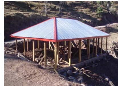
Figure 3 51. Simple frame at the start of the process of converting the posts into dhajji walls with hipped roof. Note that gutters are not provided to any of the roofs. (Note: This is an early stage construction photo. There are now many houses with gutters either for water or to control splash, and a big programme to increase rainwater harvesting.)
