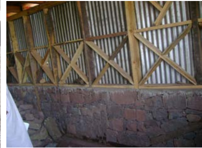
Figure 3 48. Mixed construction form. Dry stone wall with dhajji timber frame on top but without traditional infill material. Note: This is only a stage in construction. This is always infilled later. The corrugated galvanised iron sheets will be used as permanent shuttering / weather protection.
