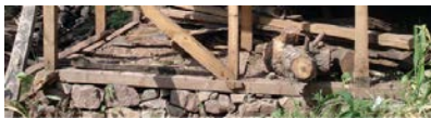
Figure 3 11. Post and plinth beam (called dassa locally) connection details. Note that the timber frame is founded directly on stone which will help keep the timber dry. (Note: The recommended way to fix the dassa is to use a small amount of concrete and some large stones to fix the bolt in place below ground then use dry stone above ground to drain properly. Focus should be on good stable plinth construction as much as the fixing.)
