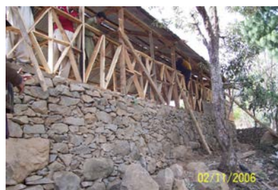
Figure 3 54. Dhajji frame built on a poor quality dry stone wall.
