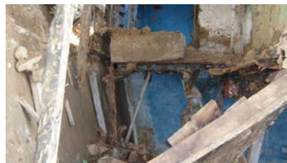
Figure 3 21. Collapsed timber floor structure of an abandoned house in Simla, India. (Note: Layer of mud laid on floor structure).
