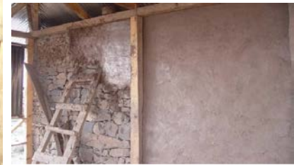
Figure 2.6. Plastering with cement sand plaster or mud mixed with natural fibres (note that the wall is not a Dhajji wall).
