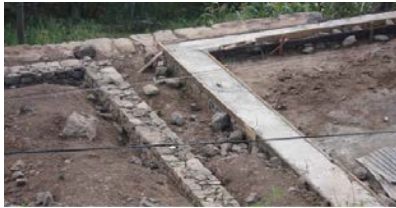
Figure 3 5. Strip footing made from stone with concrete capping and embedded steel reinforcement.
