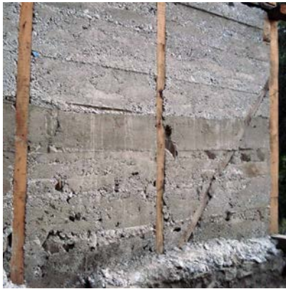
Figure 3 28. Timber, stone laid in concrete. This is not traditional dhajji construction. There is a risk that the entire panel may fall out as a rigid object during an earthquake.
