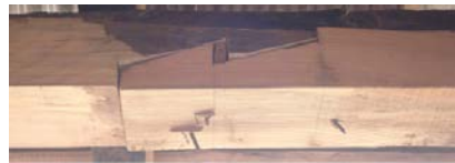
Figure 3 33. Poorly built scarf connection. The joint is a poor fit and the wooden peg that should pre-stress the joint appears loose. Note that the joint has been crudely reinforced with nails.
