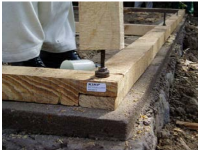
Figure 3 8. Bolting of plinth band with foundation. Note that a damp proof course has not been used.
