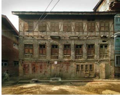
Figure 1 4. A building with Dhajji in upper most storey only from Srinagar, India. Photo source: © Randolph Langenbach (see Ref. 2).
