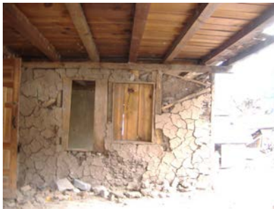
Figure 5 19. Isolated collapse of infill panel in dhajji house.
