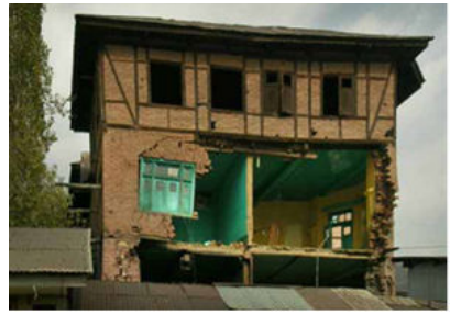
Figure 5 21. A building with dhajji in upper storey surviving although brick URM walls of lower storey toppled (Ref.: R. Langenbach, www.traditional-is-modern.net ).
