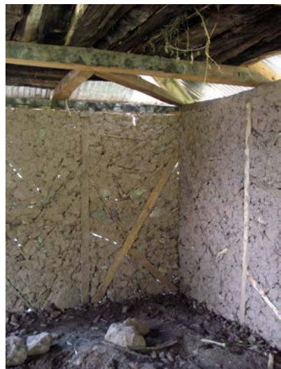
Figure 3 27. Internal view of completed wall. Note that the timber frame is not protected from getting wet as it is built straight in to the ground.
