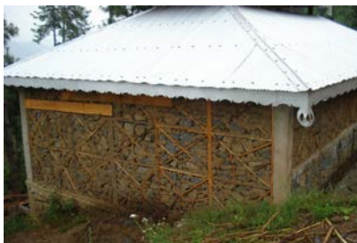
Figure 3 38. Mixed reinforced concrete and timber framing in dhajji style using X-bracing pattern.
