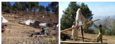
Figure 6 4. Cutting of timber sections with the help of motorised saws is rarely available. Old fashioned labour is more common, especially in more rural settings. Note: Motorised saws travel to sites on hire and this is becoming more common.
