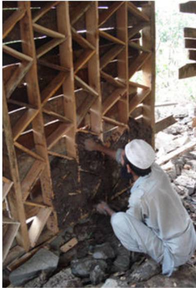
Figure 3 14. Construction of wall with stones and mud mortar. The planks on the other side of the wall act as formwork and will be removed after the infill placement is completed.
