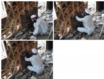
Figure 6 13. Construction of the infill walls continued. Note: Note he was breaking the stones as he went along. Previously large stones from an old unreinforced stone house on the same site.
