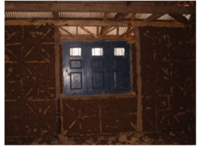
Figure 3 15. A wall ready to receive final coats of mud plaster (view taken from inside a building).
