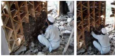
Figure 6 11. Construction of the infill walls. Note the very thin timber section sizes being used for both vertical and zigzag bracing pieces.
