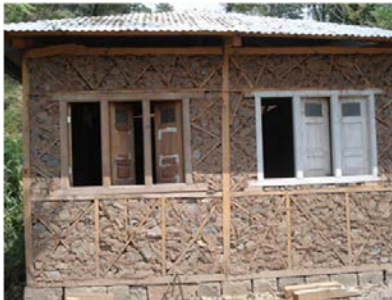
Figure 3 17. A completed wall. Note that the entire building has been raised above the ground level by a stone masonry foundation.
