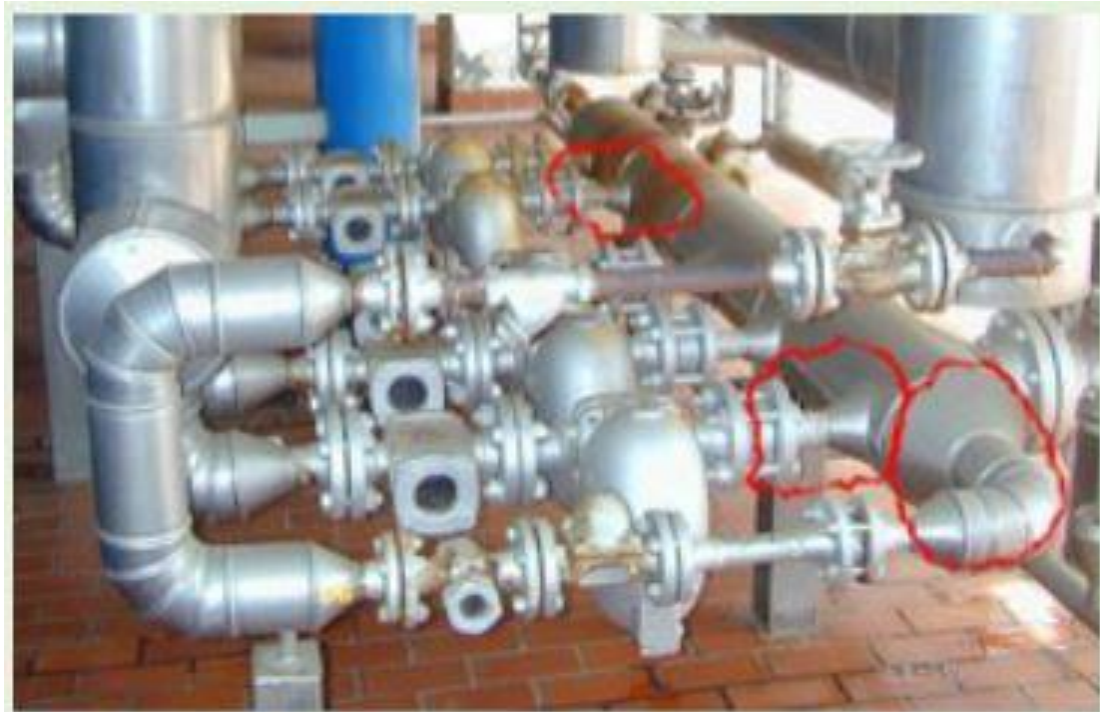
Steam Trap Installation
