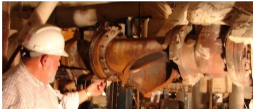
Blown out Strainer upstream of 120 psi PRV Station that was being re-energized after a brief shut down for maintenance
