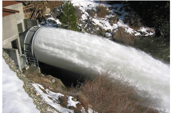
Salt River and Lower Bear Reservoirs, California, USA—Four Howell-Bunger® Valves, with stationary hoods (18", 24", 60", 78")
