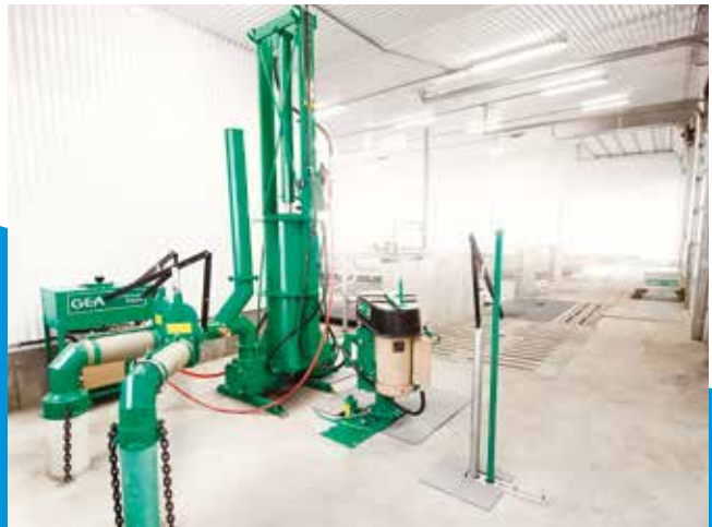
Electromix system on the floor above the reception pit. Installation with double discharge for manure transfer in two different pits.
